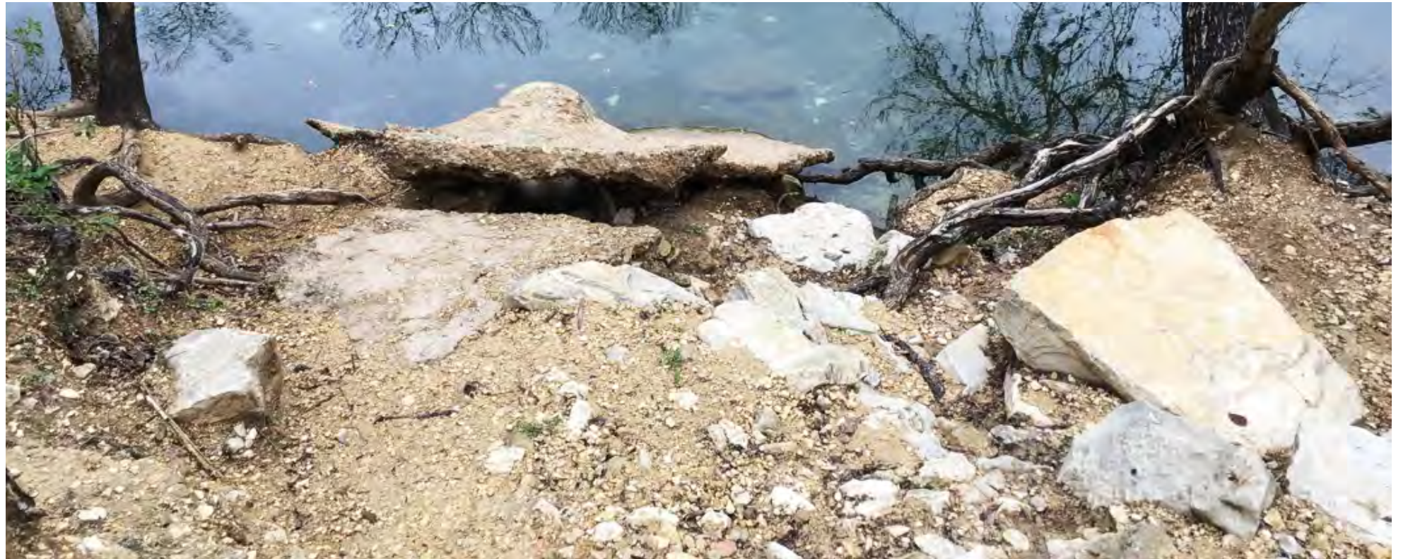
Decomposed granite decomposition near water edge
